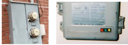
Figure 5 Energy monitors (left) Geraldine uses her energy meter as a monitoring device to let her know how much energy she is using. (right) An “Energy Saver” device that Jacqueline uses to help determine how much energy she’s using. For Jacqueline, the device specifies three colors: Yellow = “Caution”, Green = “green light is fine” and Red = “You’re getting a light bill”
